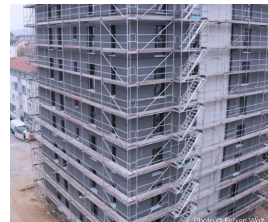
Pictures below: Development of a multi-story construction by B&O Bau in Fürth.
